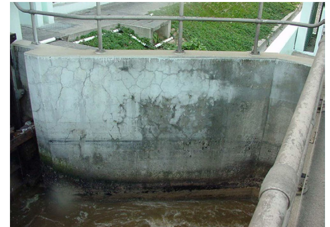
Shek Wu Hui Treatment Plant, cracks identified in 1991
